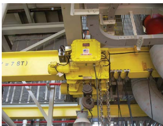
SPARK RESISTANT/EXPLOSION PROOF, 10-TON CHESTER LOW HEADROOM ELECTRIC CHAIN HOIST IN USE ON AN OFFSHORE OIL PLATFORM.
